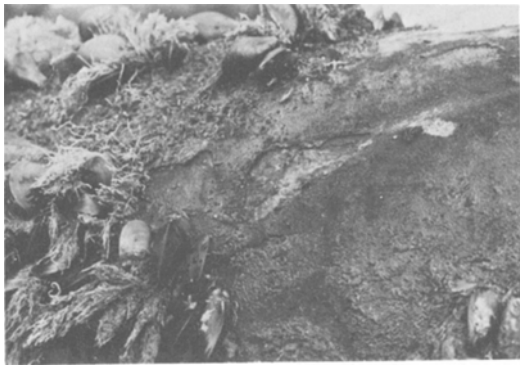
Figure 6 Example of enhanced corrosion on cathodically protected structural steel below marine fouling.
